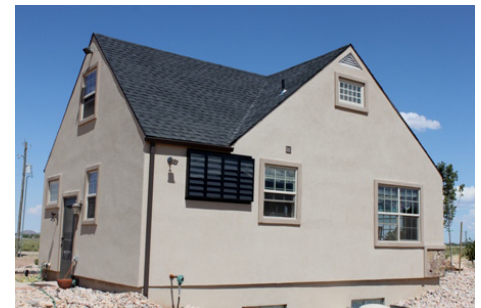
Wall mounted solar hot air collector. Source: www.solarairsystems.com
