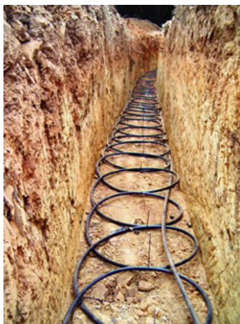
Horizontal loop field photo credit: Air Solutions
