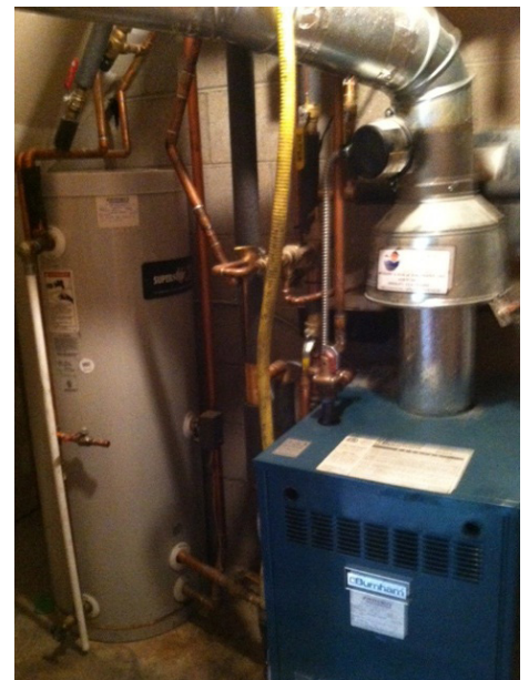
An indirect water heater: the blue boiler heats water in a pipe that runs in a coil through the storage tank for both space and domestic hot water heating.
