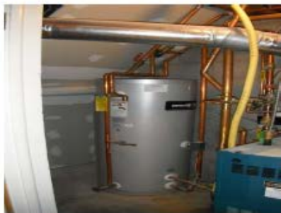
Your Water Heater
