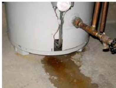
Leaking Water Heater
