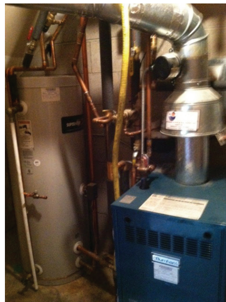
An indirect water heater: the blue boiler heats water in a pipe that runs in a coil through the storage tank for both space and domestic hot water heating.
