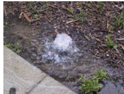
Figure 3: A broken sprinkler head wastes water.
