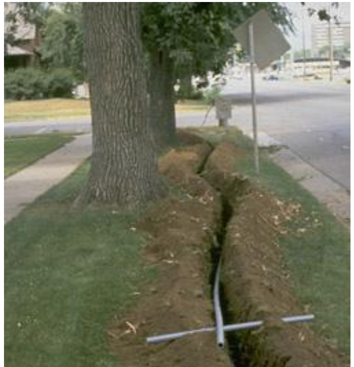
Figure 5: Trenching near trees can severely damage root systems.
