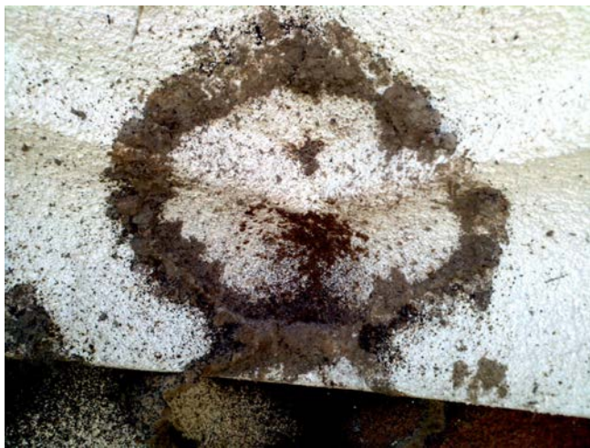
Figure 10. Area of a cliff swallow nest after it has been removed. In the center of this photo is a cluster of many dozens of swallow bugs. Later these will scatter for cover and may find ways to enter interior areas of the building. Photograph by Brandon Ewals-Strain.
